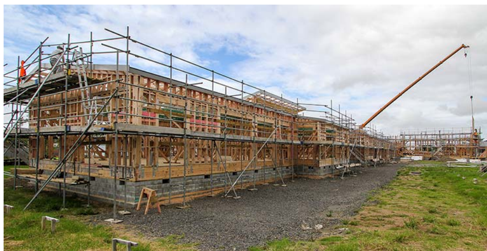
• Work is well underway on the new seven classroom block - the new hall is in the background
