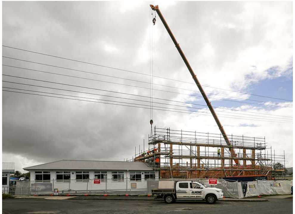
• A giant crane lowers a wall panel into place between the new hall and the relocated library
