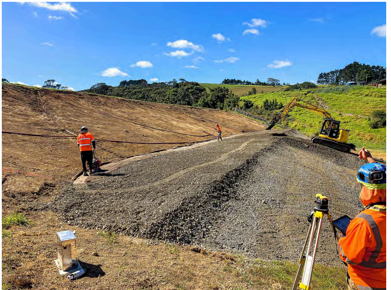
• Placing and levelling of the Mangakura Dam 1 embankment fill layer as part of the $3m upgrade
